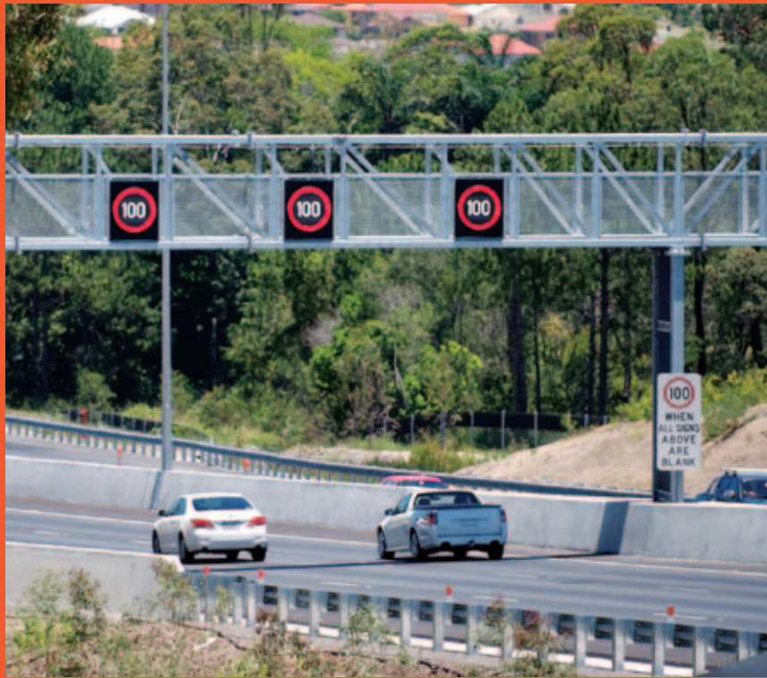
VARIABLE SPEED SIGNS LOCATED ON THE GATEWAY MOTORWAY.
